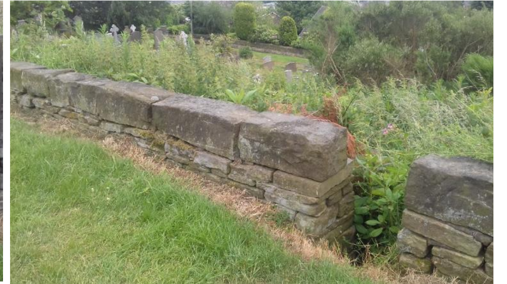
Photo 9: Gap in wall onto 'Moss Side' half way between point A and point E 22/6/2017
